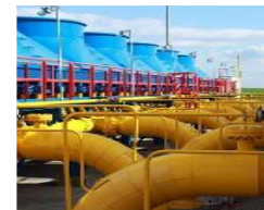
Petroleum and petroleum products pipeline transmission or distribution systems
