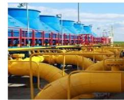
Petroleum and petroleum products pipeline transmission or distribution systems
