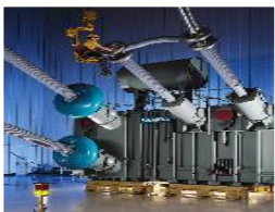
Distribution of electricity
